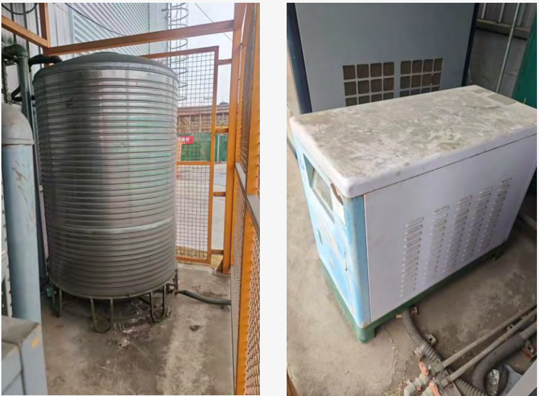
▲ Waste heat recovery equipment
